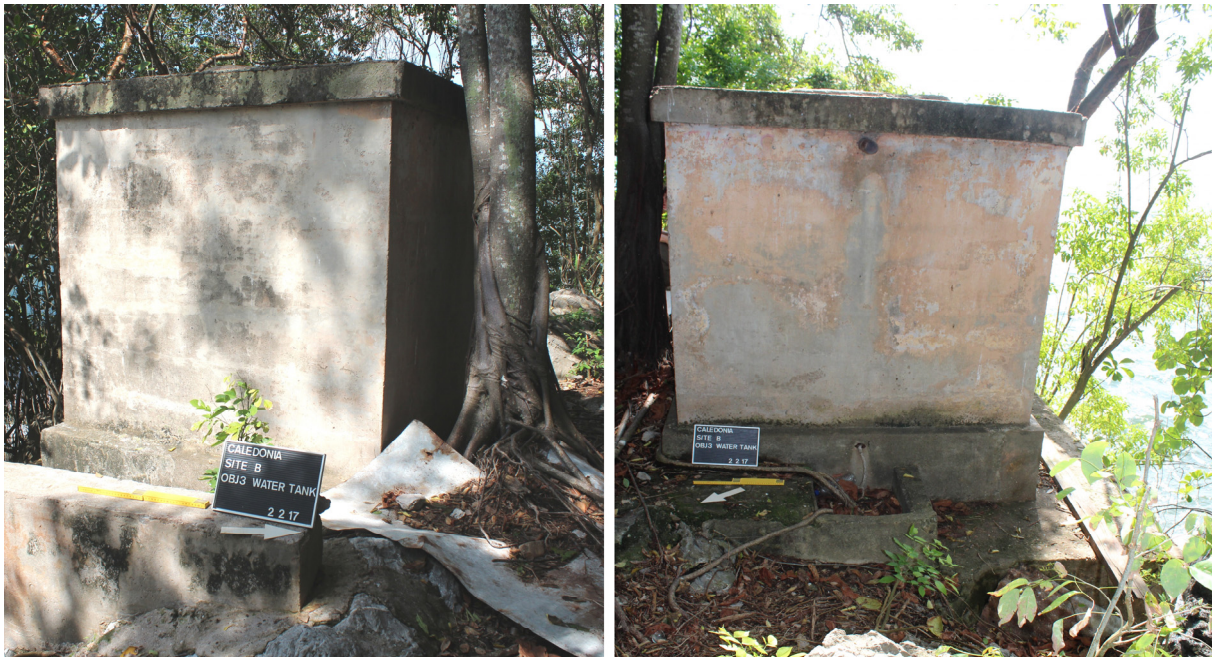
Figure 7: Water Tank as seen from a) the east and b) the north-west, showing the pipes and basin
